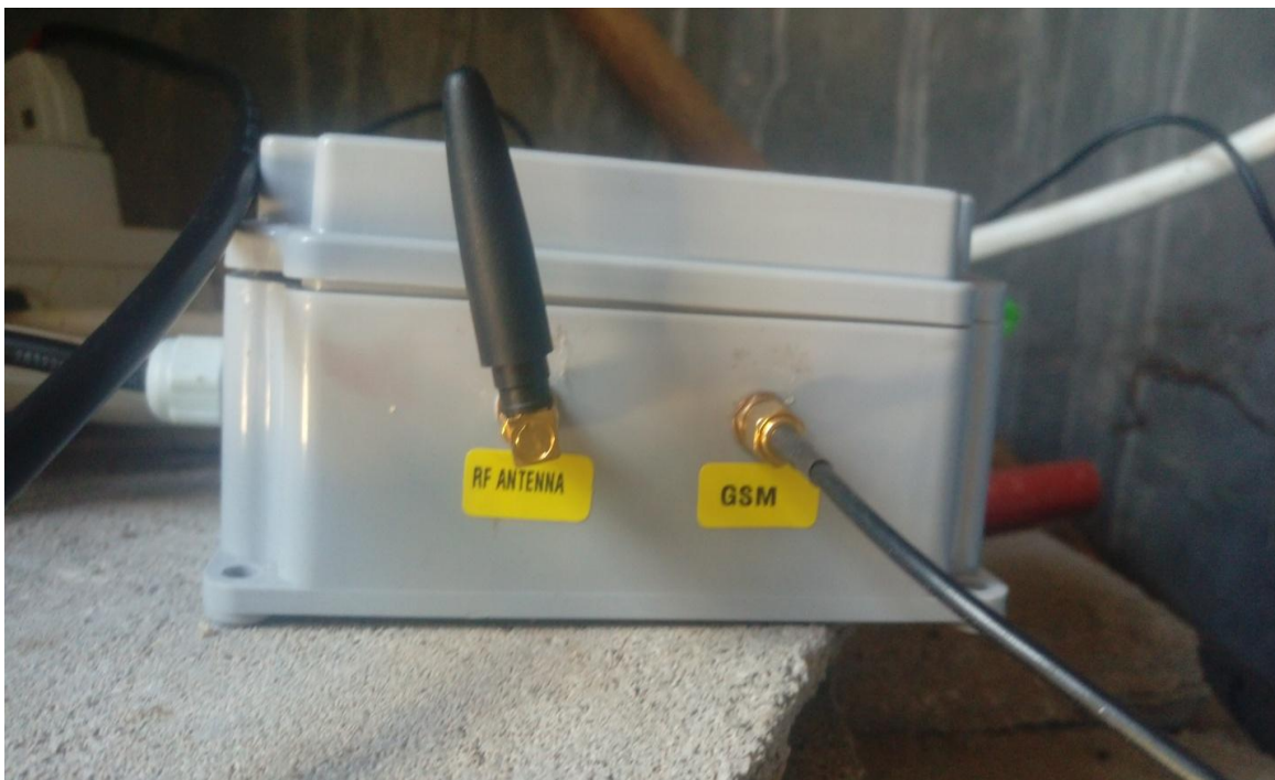
Figure35: Gateway Router Interfaces-GSM and RF Interfaces
